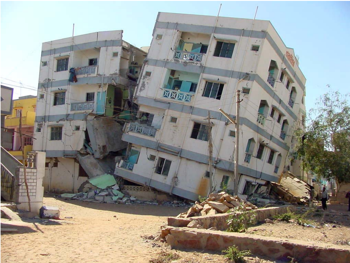
Figure 4.25: Weak storey in a building: collapse of open storey in the five-storey residential building during 2001 Bhuj earthquake (India) in Bhuj town
