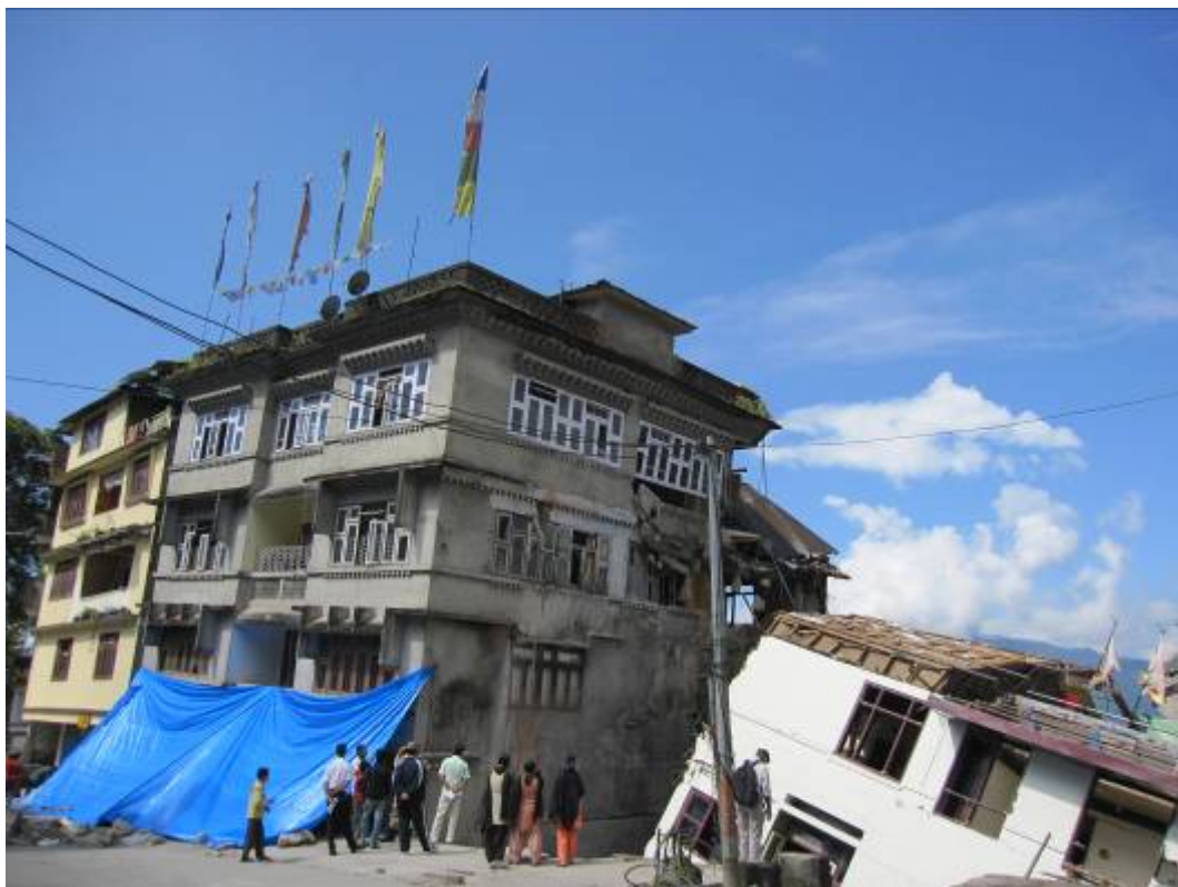
Fig. 7. Collapse of two multistory RC frame buildings at Balwakhani, Gangtok (Photo: Tripti Pradhan)
