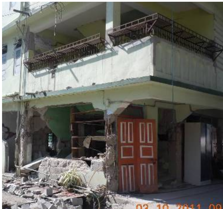
Fig. 12. Complete damage of columns and exterior wall in a building at Chungthang due to poor detailing of column reinforcement, lack of confining reinforcement, improper splicing of rebars, inferior detailing of columns with corbel (Photo: Tripti Pradhan)
