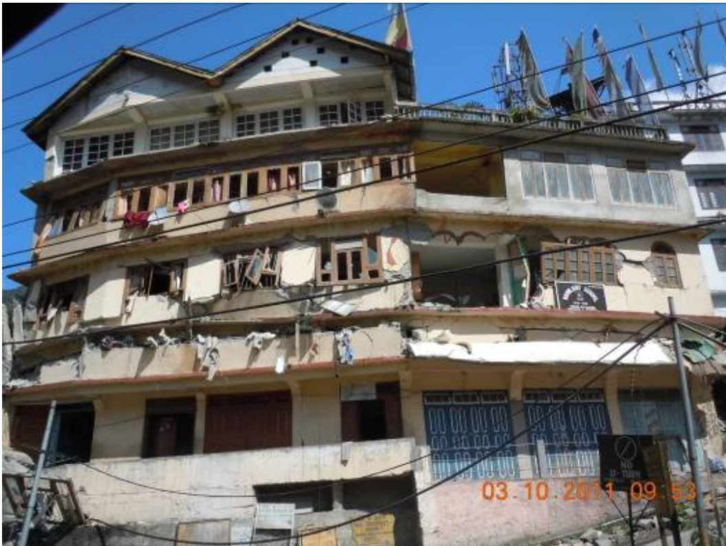
Fig. 11. Pancake collapse of the third storey of the five storey school cum residential building in Chungtang (Photo: Goutam Mondal)
