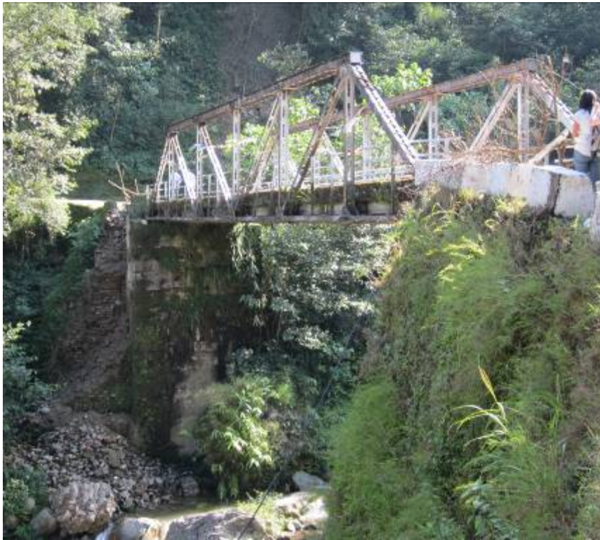
Fig. 15. Damage to the wing wall of steel truss bridge on Raykhola (photo: Tripti Pradhan)
