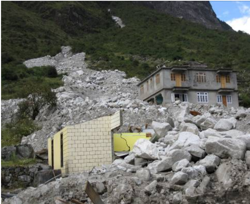
Fig. 6. Damage due to rock slide after two days of the event in Lachung (Photo: Neha Parool)
