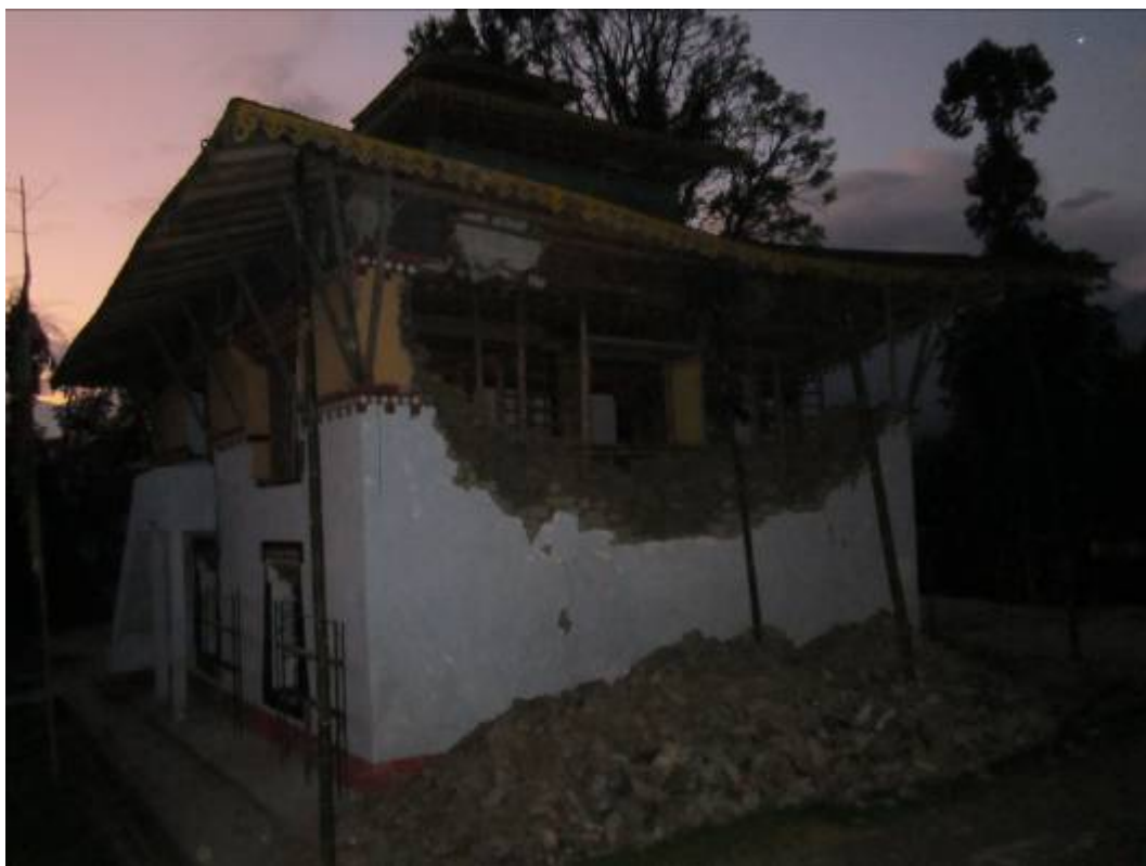
Fig. 18. Partial collapse of stone masonry walls of a Monastery temple at Mangan (Photo: Goutam Mondal)
