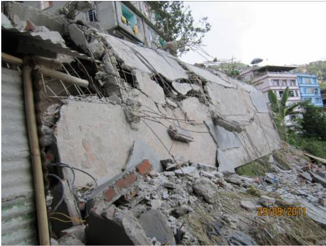
Fig. 10. Complete collapse of newly constructed RC building at Lumshey Basti, Gangtok (photo: Neha Parool)
