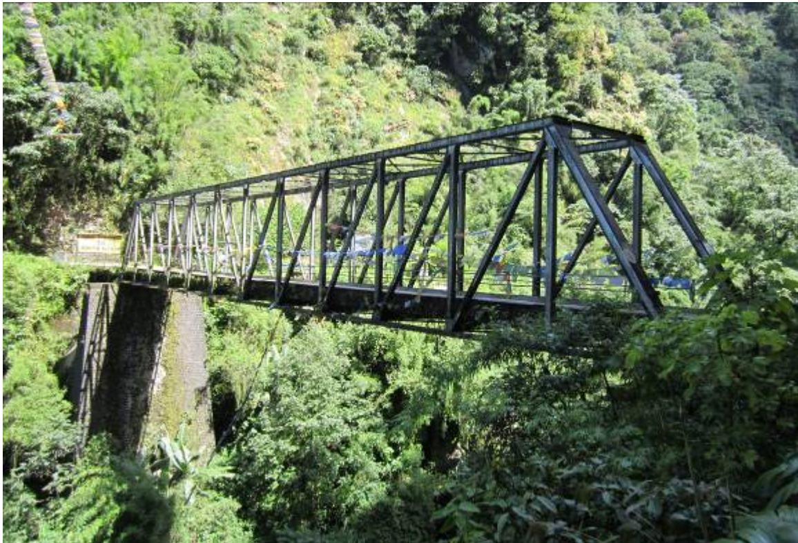
Fig. 17. Undamaged steel truss bridge connecting West Sikkim and North Sikkim (Photo: Vaibhav Singhal)
