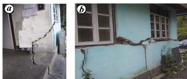
Figure 6. Damage to brick masonry houses with CGI sheet roofs. a , Subsidence due to sinking of the fill part of the foundation. b , Cracks extending up to the plinth, indicating the need for plinth beam to hold the structure together.
