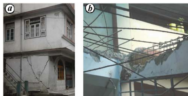
Figure 8. Damage to RC-frame buildings. a , Non-structural damage in the form of diagonal cracks in the infill walls and separation from RC frame. b , Severe structural damage to multi-storeyed, engineered school building.
