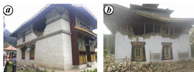
Figure 7. Extensive damage to stone masonry walls of tall heritage structures. a , Dubdi monastery, Yuksam, West Sikkim. b , Ringhim monastery, Mangan, North Sikkim.
