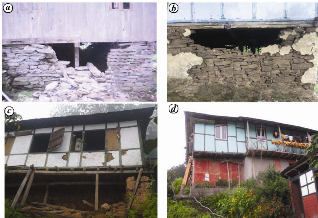
Figure 4. Partially collapsed load-bearing stone masonry wall supporting light-weight bamboo/wooden house with CGI sheet roof. a, b , House with ( a ) wooden walls and ( b ) with bamboo and wooden frame. c, d , Retrofitting with wooden posts.
