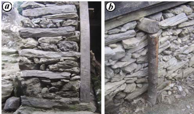
Figure 5. Cross-section of the stone masonry wall with mud mortar. a , 'Through stones' in stone masonry wall are vital in preventing the wall from collapsing. b , Bulging is more prominent in stone masonry walls because of the absence of 'through stones' and needs to be retrofitted with wooden posts.
