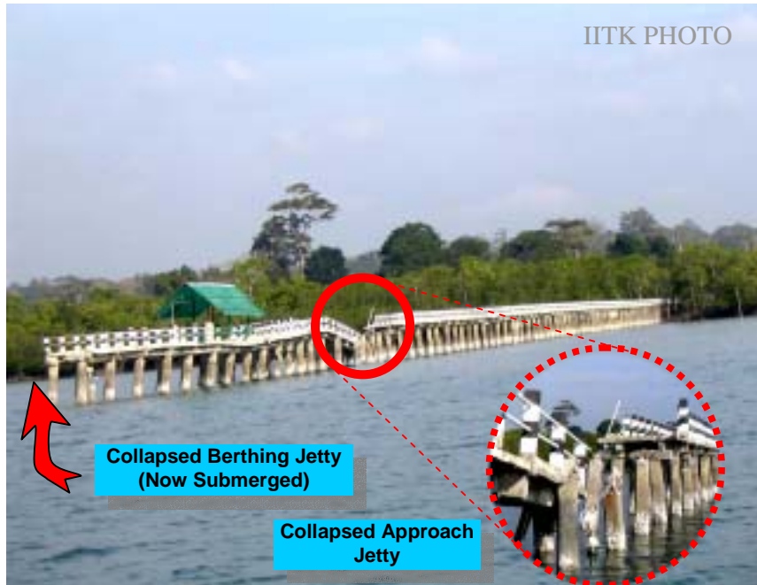
Figure 17: Gandhinagar Jetty in North Andaman: Total collapse of the berthing Jetty and partial collapse of the approach jetty. (Photo: Durgesh C Rai)
