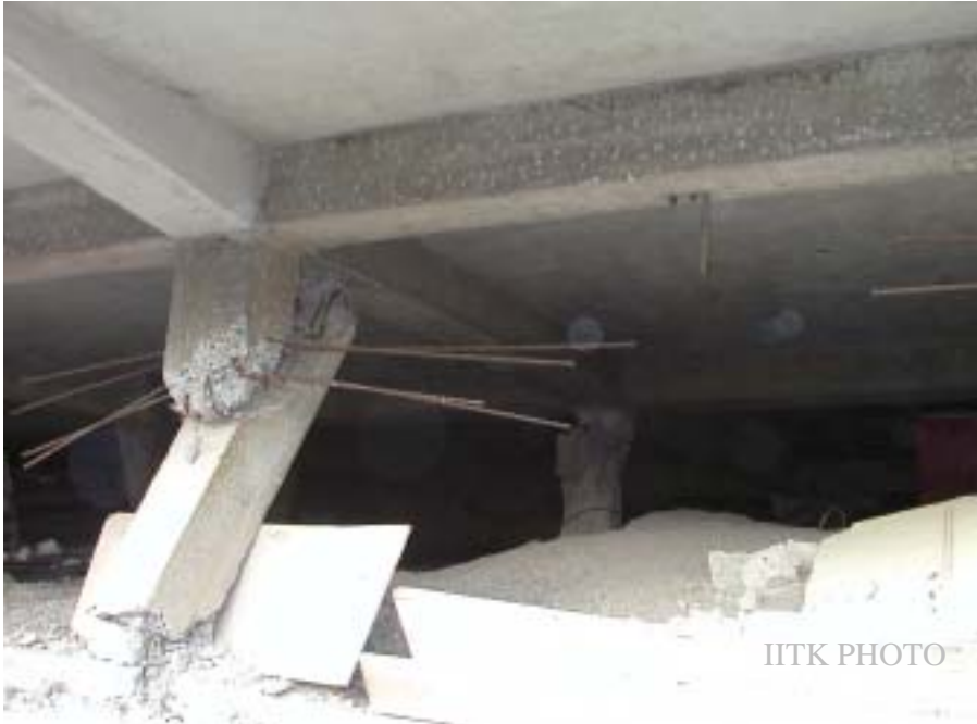
Figure 11: Collapse of a three storey reinforced concrete frame building at Port Blair (Photo: Sudhir K Jain)
