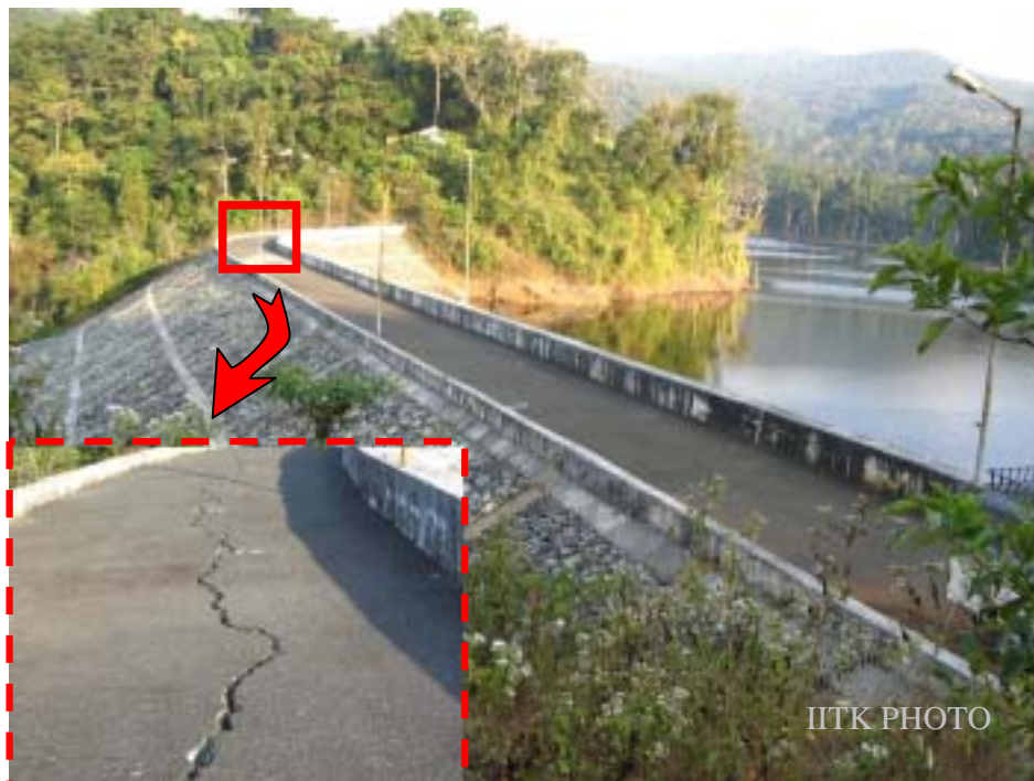
Figure 20: Longitudinal cracks at the crest of rockfill dam of the Kalpong hydro-electric project near Diglipur (Photo: Goutam Mondal).
