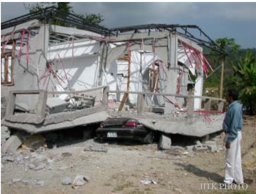
Figure 12: Collapse of a stilt Plus one storey house in reinforced concrete near Port Blair. (Photo: Sudhir K Jain)
