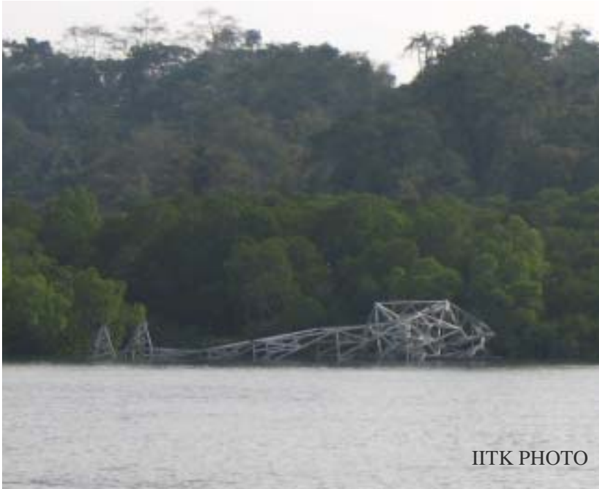
Figure 21: Collapse of electric power transmission tower at Middle Strait (between South and Middle Andaman Islands), disrupting the power supply from Kalpong Hydroelectric Project to Baratang island (Photo: Durgesh C Rai).
