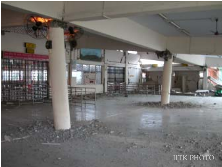
Figure 10: Severe damage to Passenger Terminal Building at Port Blair. (Photo: Sudhir K Jain)
