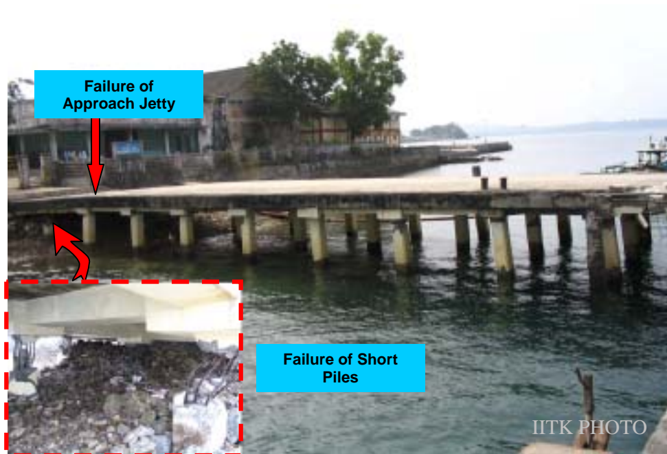
Figure 19: Shear failure of short piles of the approach jetty at Mayabandar in Middle Andaman Island (Photo: Durgesh C Rai)
