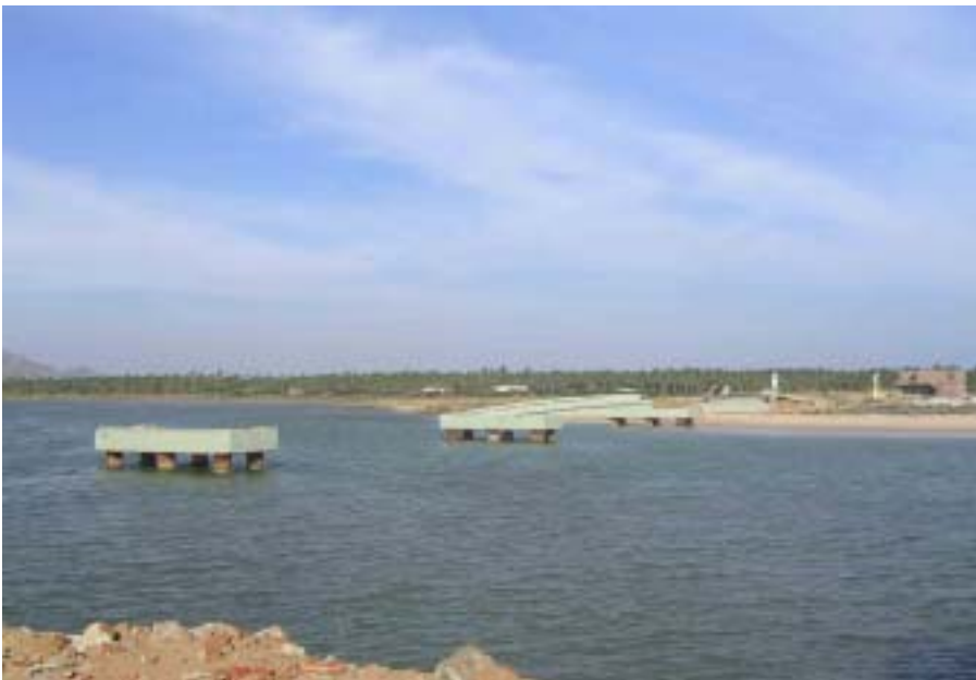
Figure 16: Complete loss of spans of the four span RC bridge at Melmannakudi. (Photo: Alpa Sheth)
