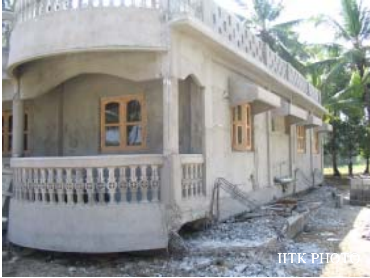
Figure 13: Collapse of an open storey reinforced concrete house at Rampur, near Mayabunder. (Photo: Durgesh C Rai)
