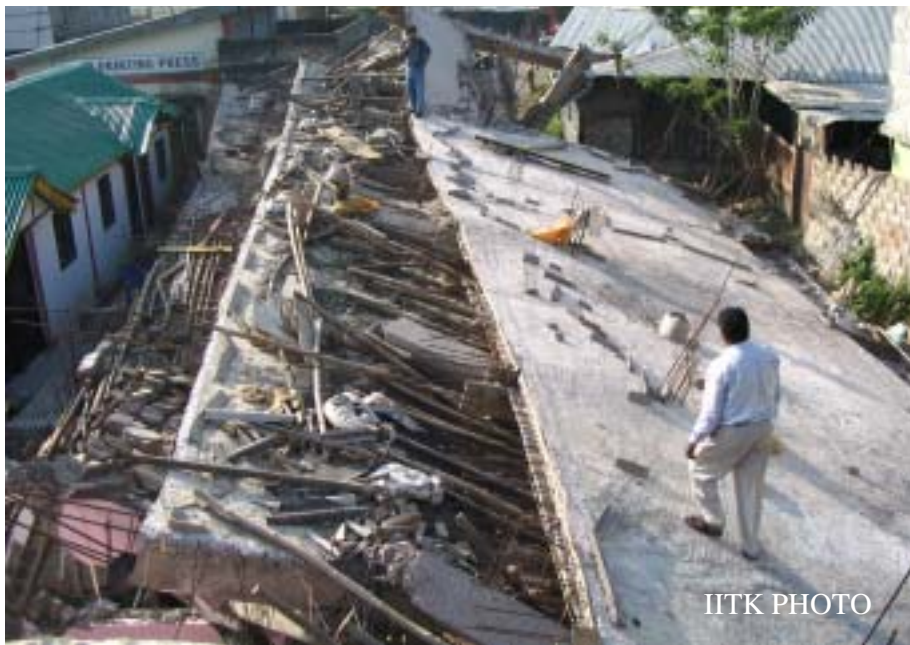
Figure 14: Collapse of RC bare frame of three storey building under construction at Rangat, Middle Andaman Islands. (Photo: Durgesh C Rai)
