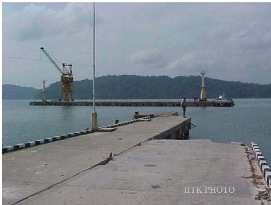
Figure 18: Collapse of the 80m segment of approach in Great Nicobar Island jetty at Campbell Bay This has adversely affected the relief work. (Photo: CVR Murty)
