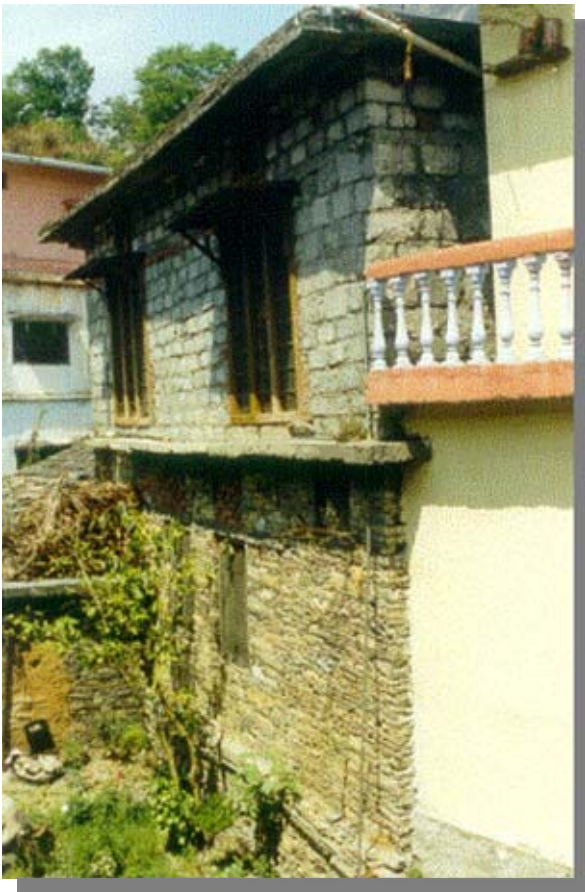
Figure 9: Two-storey house at Pipalkoti with no damage. Ground storey in slate wafer masonry, upper storey added later in concrete block masonry. Both storeys have RC lintel band
