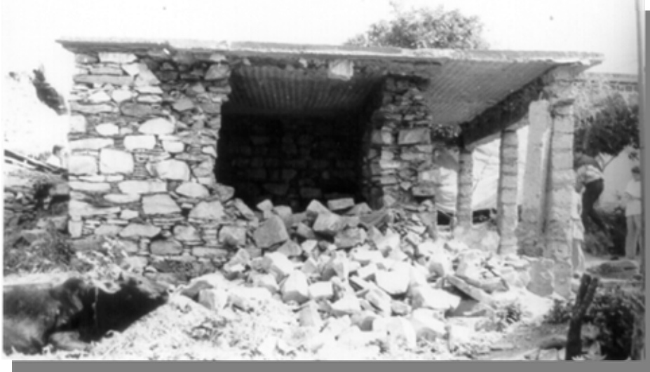
Figure 8: Partial collapse in a random rubble stone masonry. Note that the front portion has RC beam supported on concrete block columns and roof consists of RC slab
