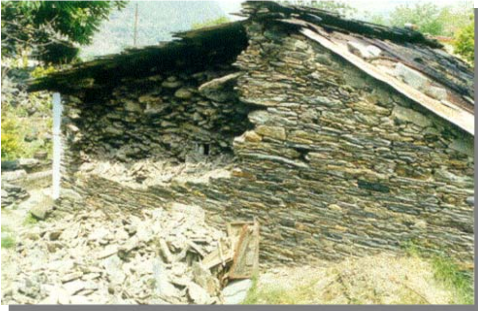
Figure 7: Collapse of one of the wythes in a traditional house in slate wafer masonry.
