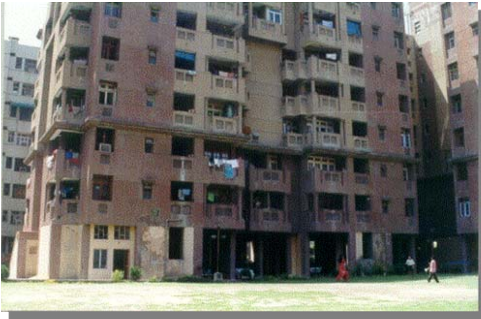
Figure 11: Tarang Apartment in Delhi that sustained damage due to infill walls
