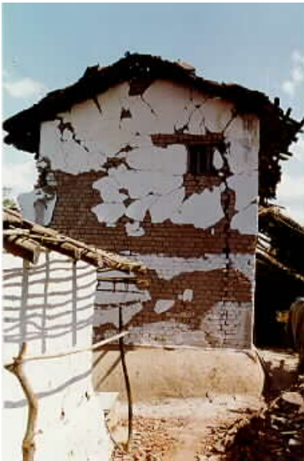
Figure 3 - In rural and urban areas, houses are built using a single wythe of burnt brick with mud mortar. Buildings of this type suffered significant cracking.
