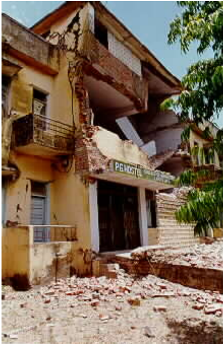
Figure 4 - Load-bearing brick masonry structures on the campus of Jawaharlal Nehru Agricultural University in Jabalpur were badly damaged.
