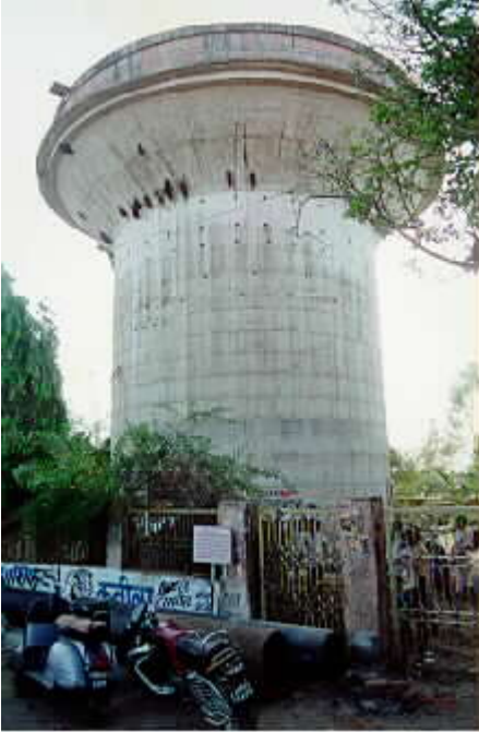
Figure 9 - Horizontal and diagonal cracking occurred at the base of the 500,000 gallon shaft-supported water tank.
