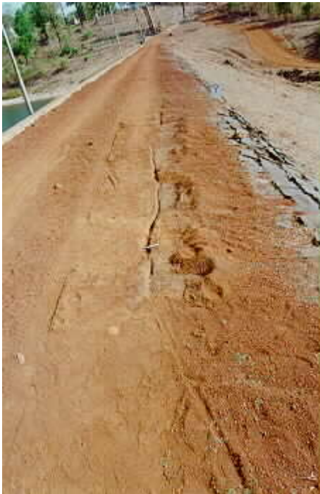
Figure 10 - Longitudinal cracks appeared along the crest and downstream face of several earthen dams.
