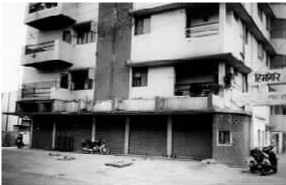
Figure 6 - The columns in the ground story parking area of the Hingiri Apartment Buildings, a five-story reinforced concrete building with brick infill, suffered shear failure.
