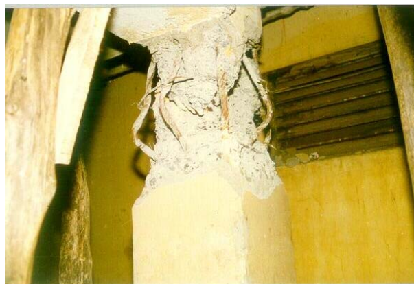
Figure 1 :: Damage to columns in Himgiri apartment.
